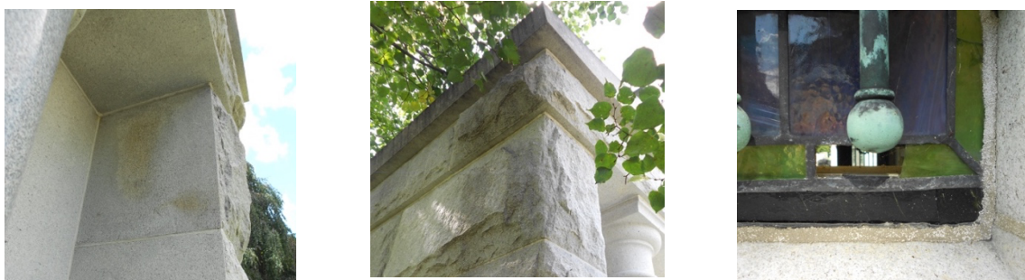
Figure 2 5 : Mausoleum Conditions (left to right)- Staining of Honed Granite, Soiling of East Façade, Missing Stained Glass Fragment
