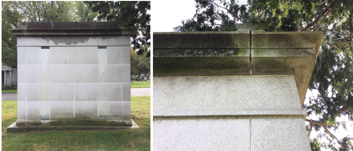
Figure 4. (left) Water remains trapped in the stone under the cornice after an early afternoon shower.
