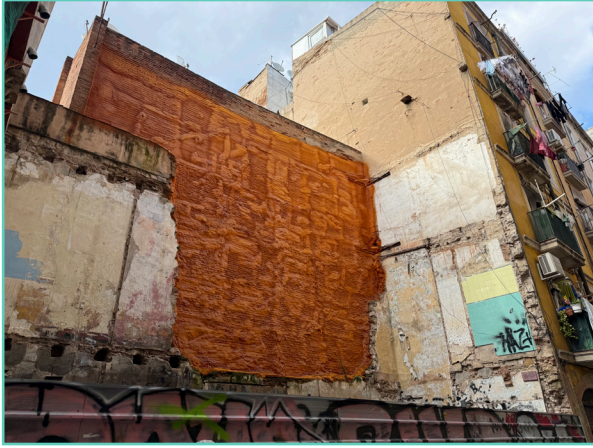
Figure 100: Building with exposed and damaged façade
