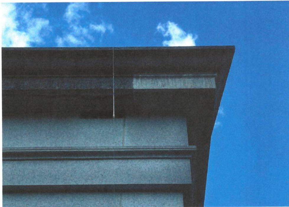
Figure 4. A clearcut starting at the jointline between the pediment and roof slab – oddly clean v.s. heavily polluted.
