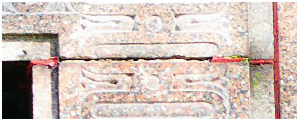
Figure 8: Areas of Mortar Loss on exterior door frame
