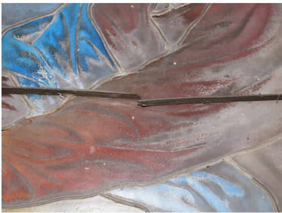
Figure 9. Photo of broken horizontal bar (second from top) on Gethsemane window.
