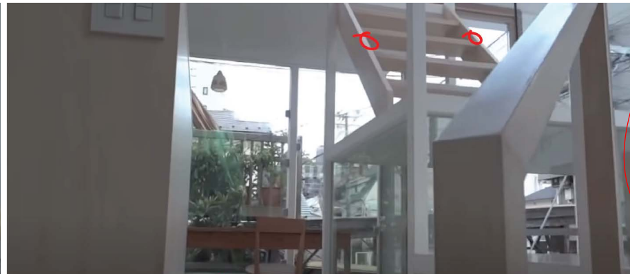
LACK OF GUARD RAILS.
