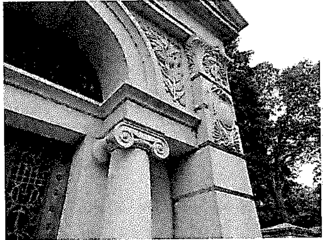
Figure 3: Granite above the mausoleum door is original, suggesting that Combs never engraved his name during construction.
