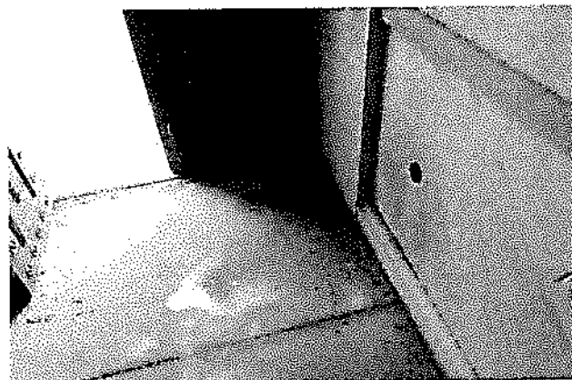
Figure 8 and 9: Water Staining at Ceiling (above); Organic Growth and Water Collection at North Corner of Interior (below)
