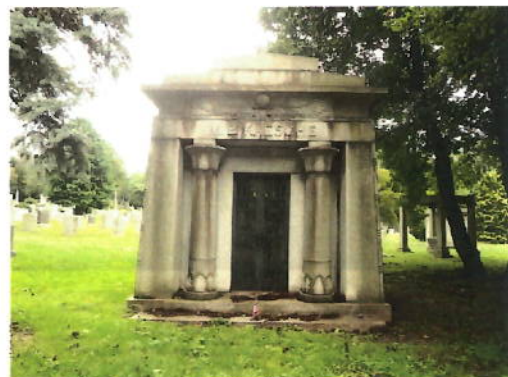
Figure 2 Front elevation of mausoleum showing Egyptian Revival Style and significant natural growth
