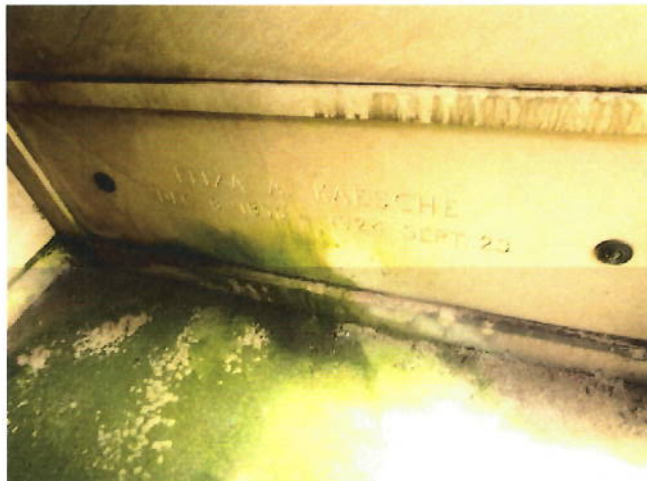
Figure 5 Interior biological growth on granite and marble surfaces.
