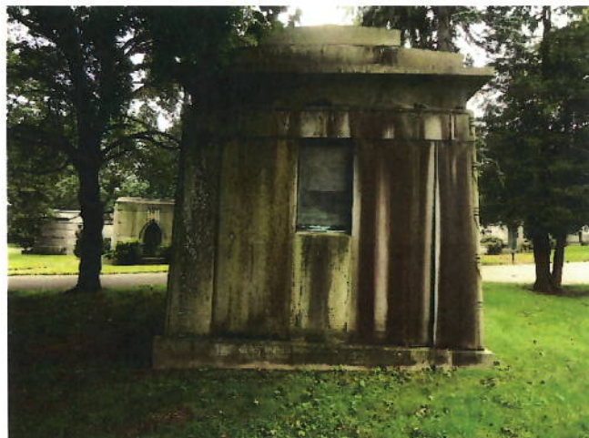
Figure 4 Biological growth on exterior facades (pictured is northeast).
