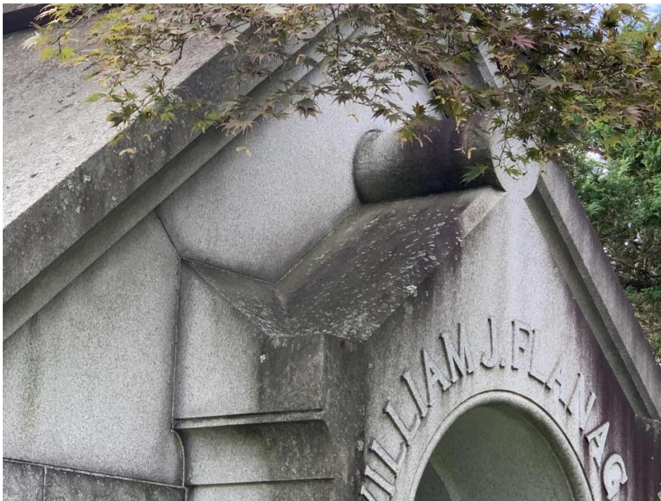
Fig.7 Biological growth on the entrance
