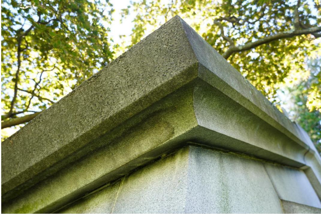
Fig.8 Biological growth around the joint
