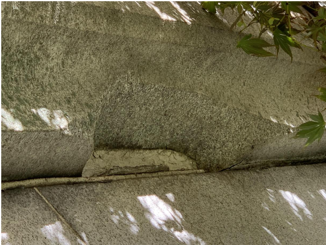
Fig.9 Spalling on the coving
