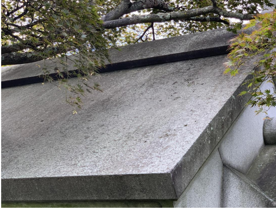
Fig.6 Biological growth on the roof
