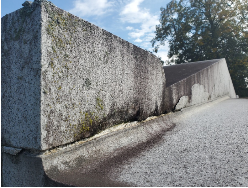
Figure G: Insipient spalling on east roof
