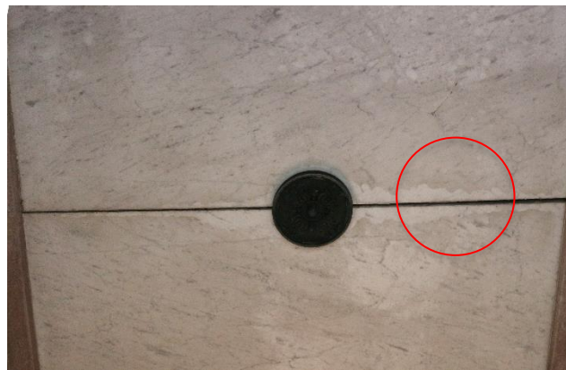
Figure 17. Gabs between the two Marble panels on the ceiling
