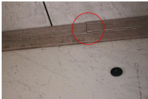
Figure 14. Cracks on the Tennessee cornice
