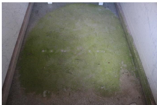
Figure 16. Biological growth on the granite floor, 2021
