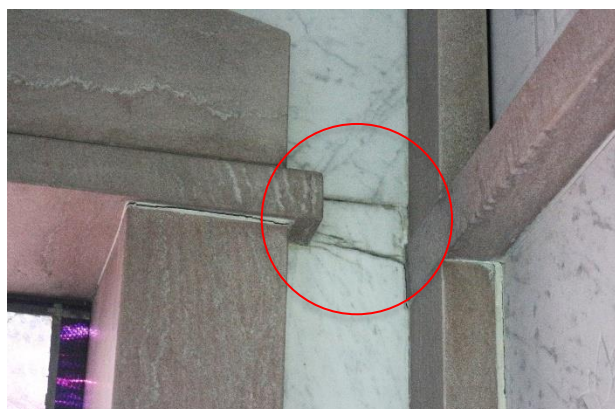
Figure 15. Cracks on the marble around the window.
