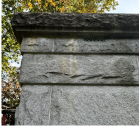
Exterior Water damage
