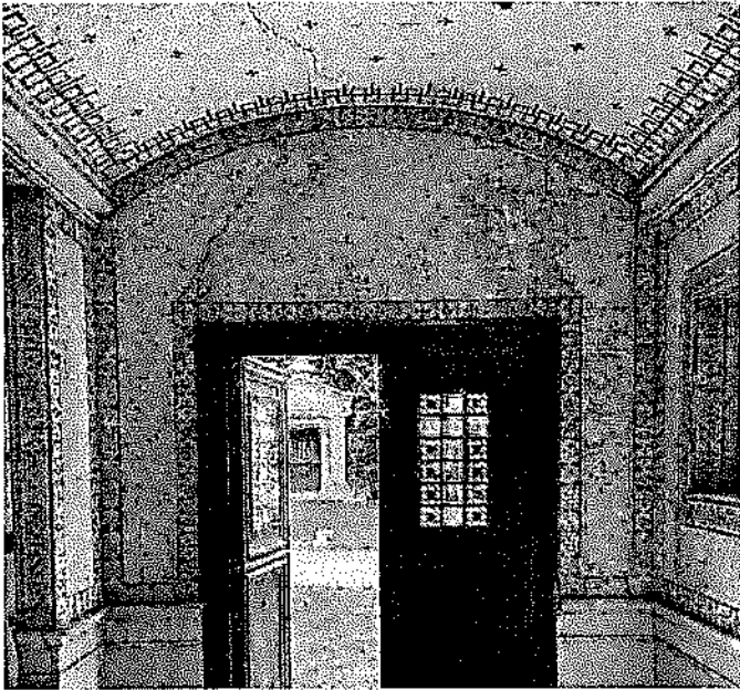
Figure 6: Front Door With Cracks
