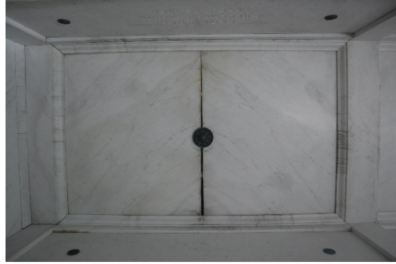
Figure 10: Gap in the ceiling that possibly caused water leakage
