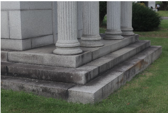
Figure 7: Biological growth in granite floor
