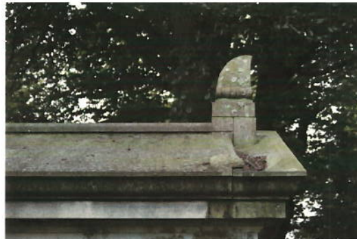
Fig 5. Detail at the roof with some water damage at the corner
