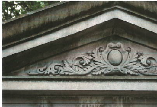
Fig 7. Salts of mortar
