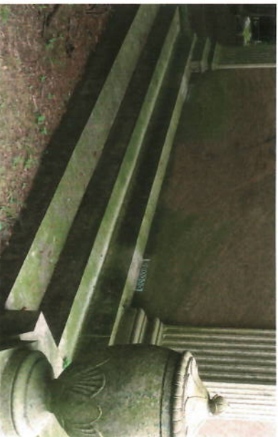
FIG. 04 DETERIORATION BY BIOLOGICAL GROWTH
