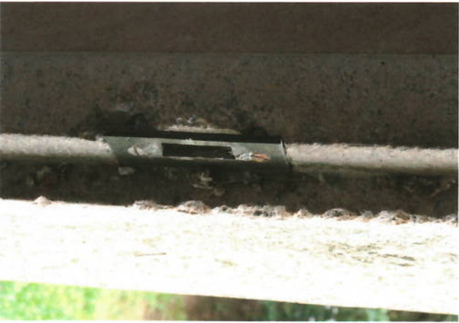
FIG. 04 DOOR JAMB CONDITION NEAR HARDWARE
