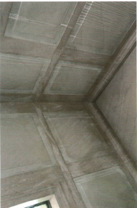
FIG. 03 WATER DAMAGE ON INTERIOR FINISH
