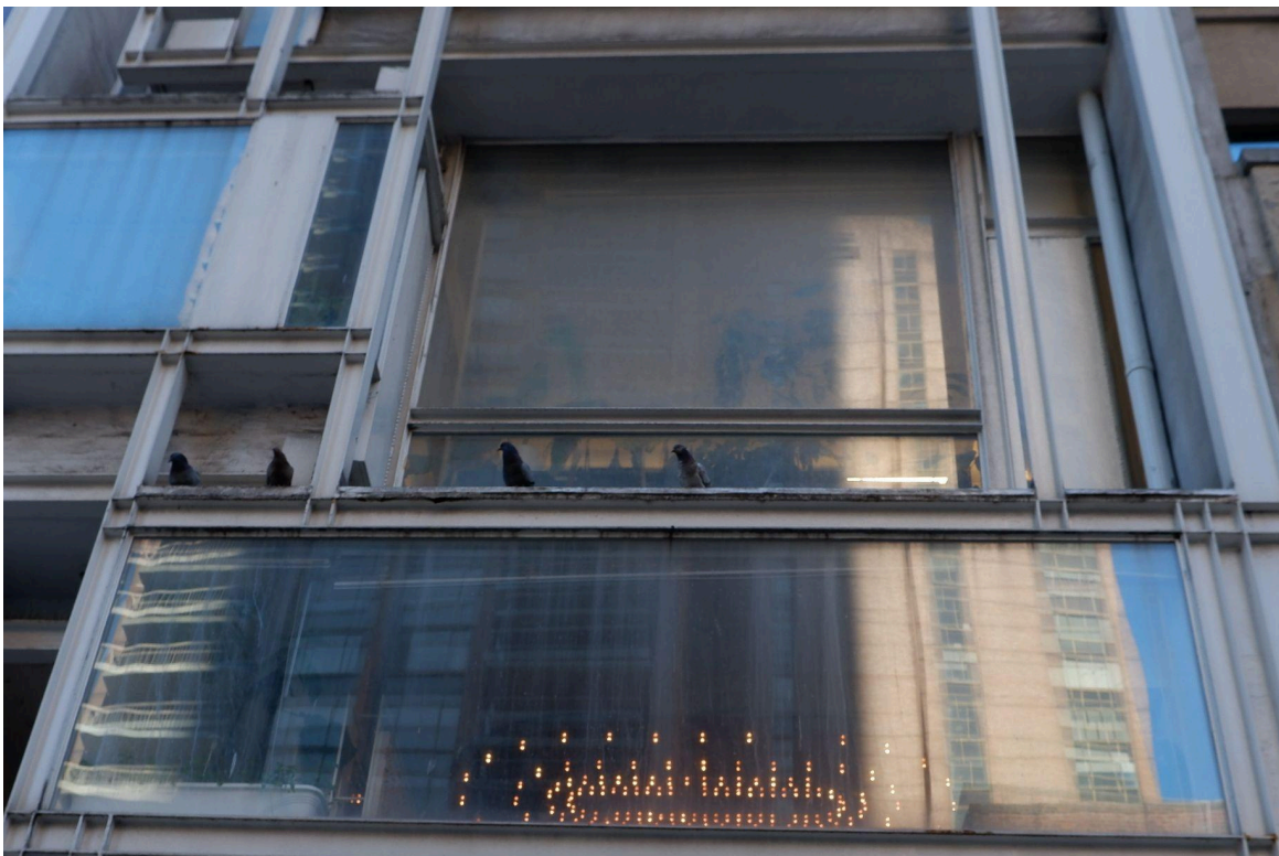
Significant patterns of soiling resulting in the displacement of roofing material occur on the setbacks found throughout the facade. This is further exacerbated by the presence of pigeons, who like to perch along the exterior. Photos by Cecelia Halle
