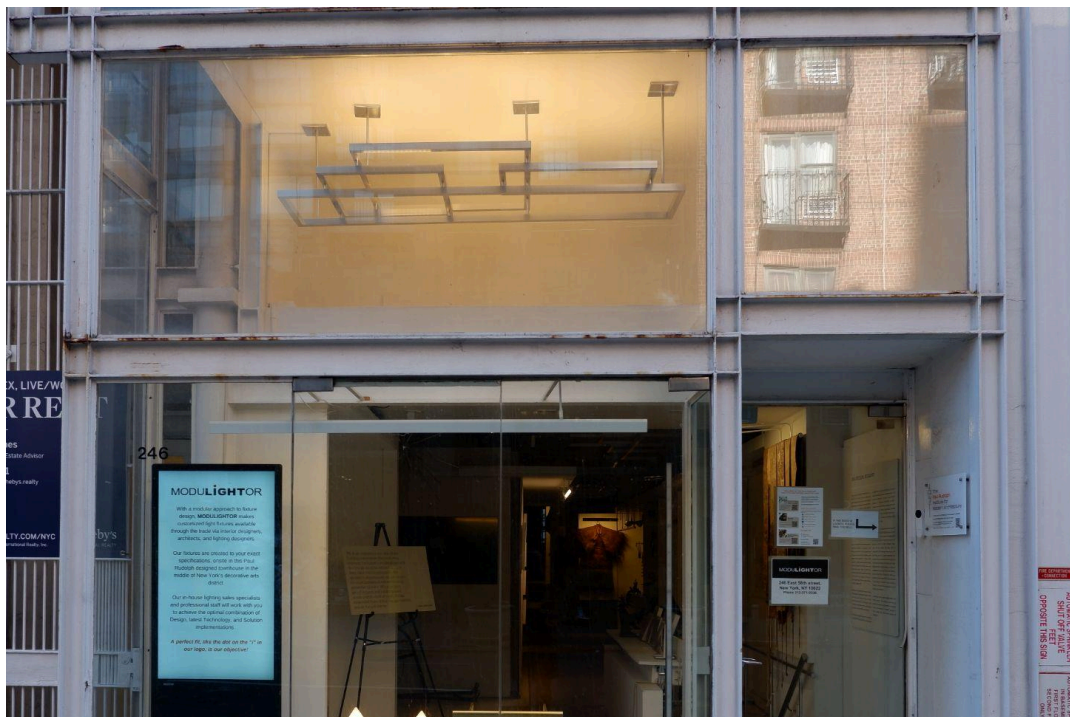
Corrosion patterning on the ground floor exterior. Photo by Cecelia Hall
