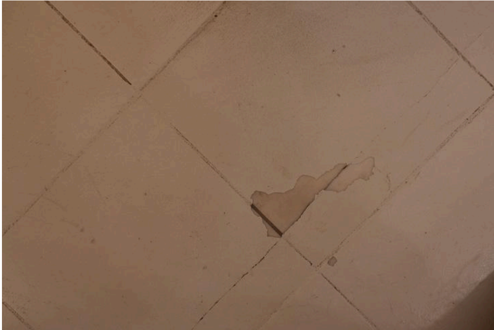
Overpainting of the flooring is also a fundamental issue throughout the interior. Photos by Cecelia Halle
