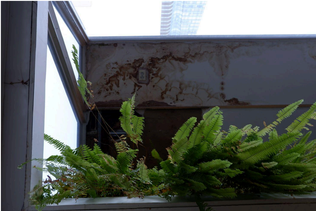
Water infiltration from the roof of the greenhouse balcony has contributed to significant surface loss, water damage, and corrosion.
