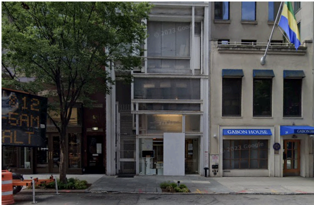
In the summer of 2022, rust jacking led to the displacement of a window pane on the entry of the Modulightor building.
