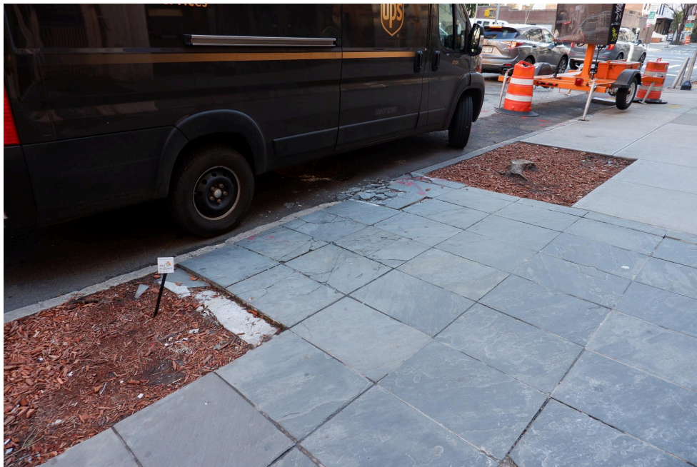
The interior grade slate that has been used to pave the sidewalk has begun to break.
