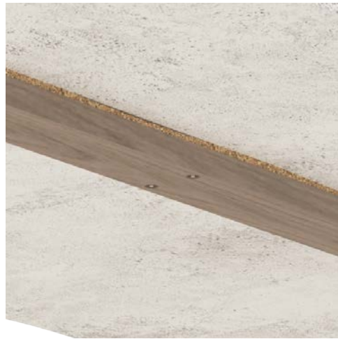
Wooden guide rail and slab anchor
