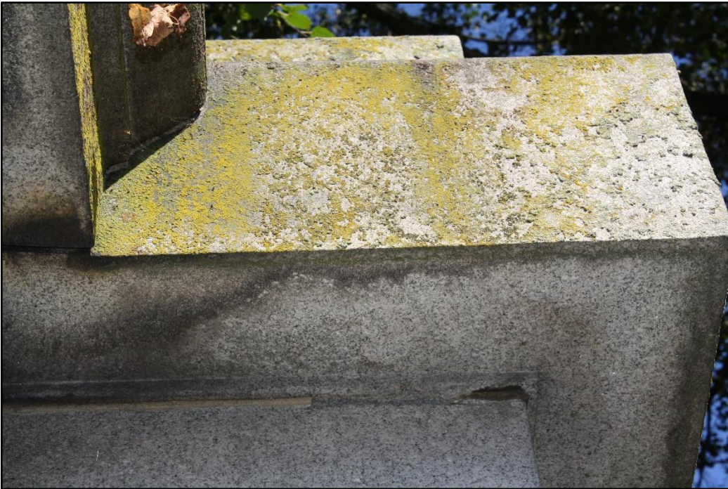
Figure 27: Biological growth located on the banding.
