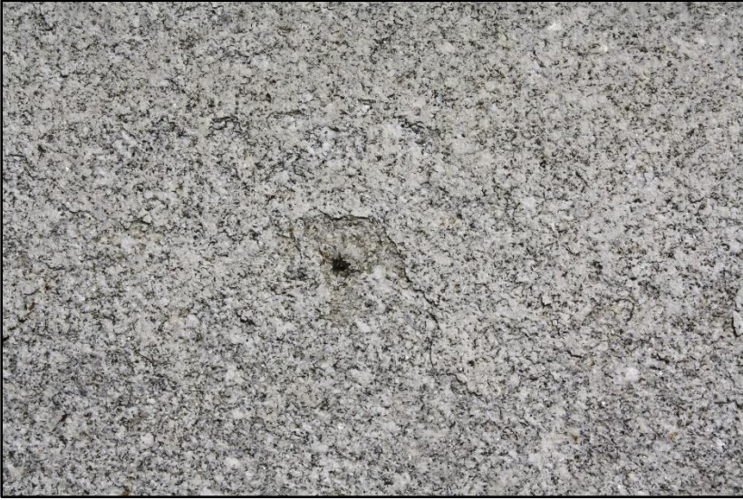
Figure 23: Close up picture of blistering and flaking marks on the exterior granite.
