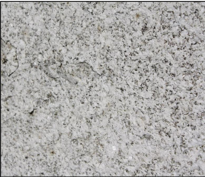
Figure 24: Second close up picture of blistering and flaking on the exterior granite.
