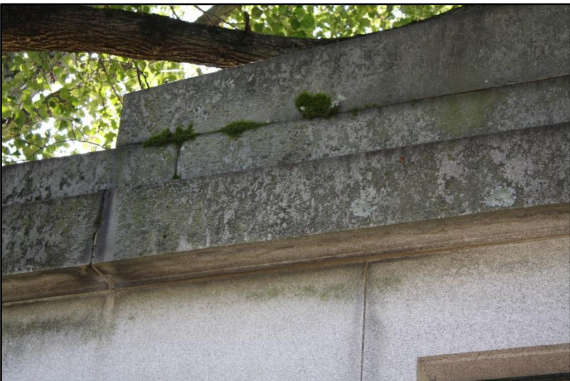
Figure 25: Biological growth located on the roof of the mausoleum.
