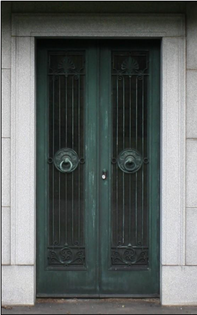
Figure 13: Fillet banding around the doorframe.
