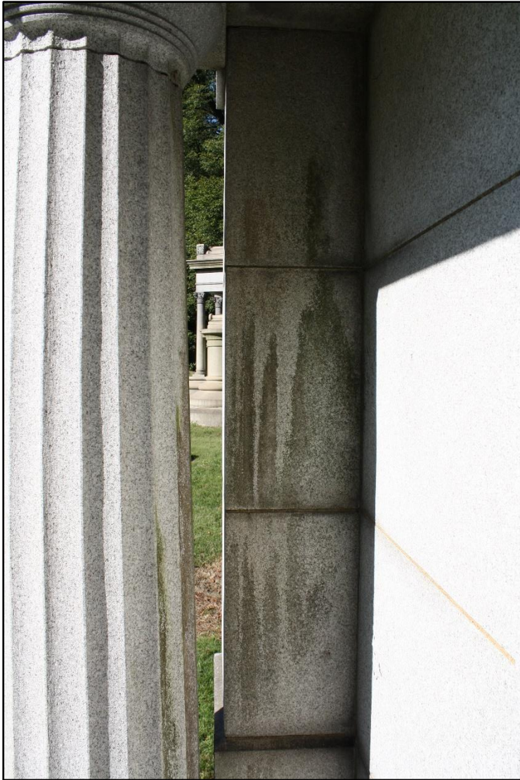
Figure 28: Biological growth located on the interior of the portico and column.
