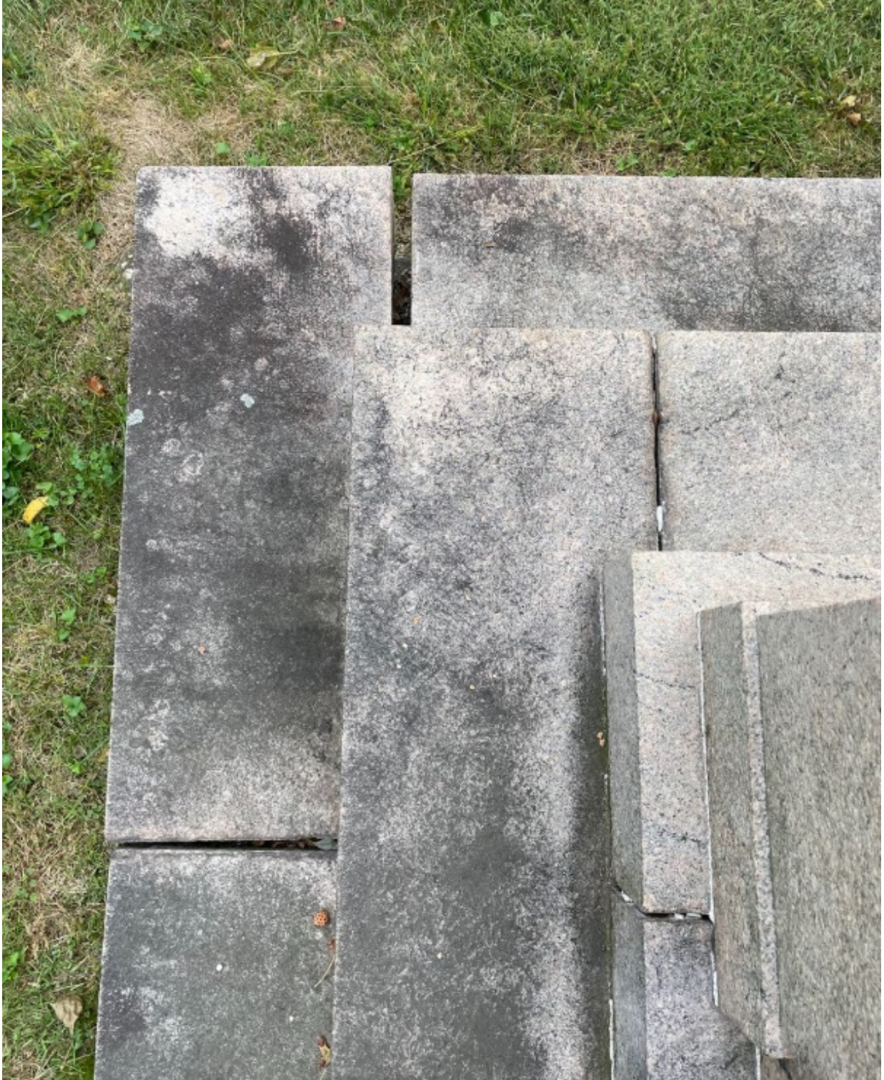
Figure 4: Southwest Corner: Lowest level step askew without mortar
