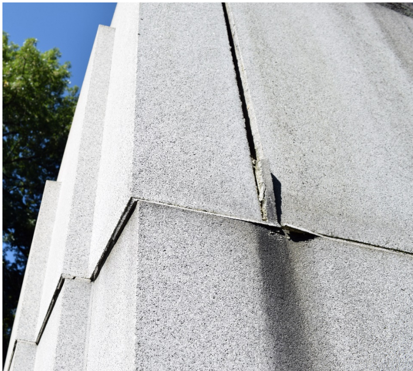
Figure 19: Widened joints on South Corner
