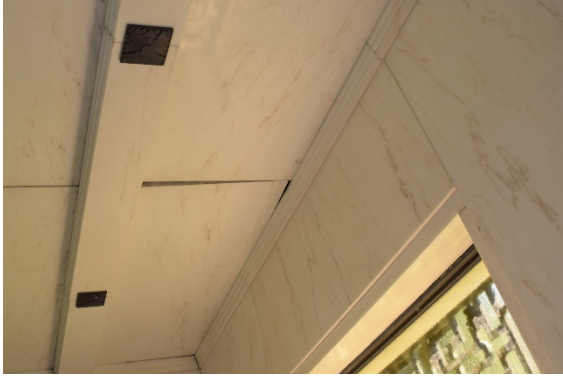
Figure 24: Displaced cladding on ceiling
