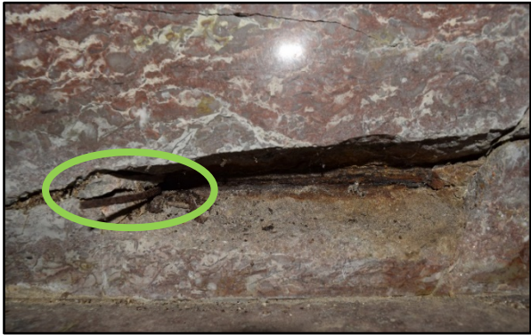
Figure 23: Cracking baseboard with rusting metal (circled)
