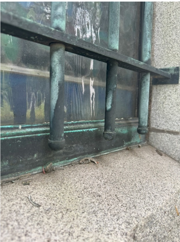
Figure 11: Degraded Seal on Exterior of Stained Glass, author's photo.
