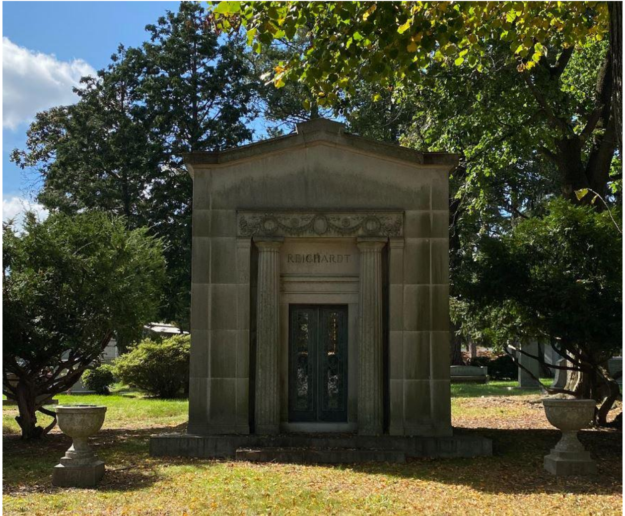
Figure 6. Water Markings on Northeast Facade
