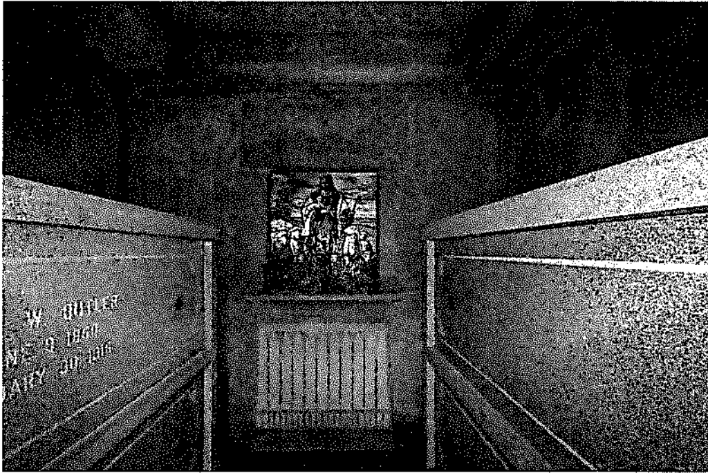
Fig. 13 Wet patches around the upper back corner joints.
