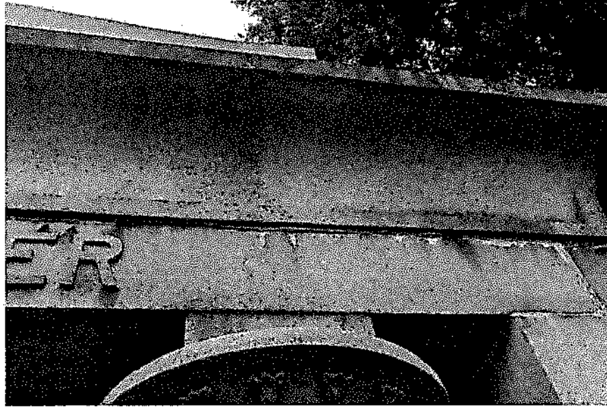
Fig. 8 Calcite deposits and rust-colored staining.
