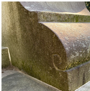
ELEMENT: COLUMN BASE CONDITION: MOISTURE / ORGANIC GROWTH AND EROTION
