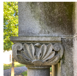
ELEMENT: COLUMN CAPITAL CONDITION: MOISTURE AND EROTION
