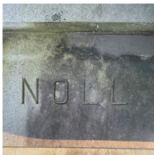
ELEMENT: STEP CONDITION: MOISTURE AND EROTION
