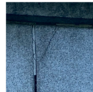
ELEMENT: MASONRY BLOCK CONDITION: CRACKING
