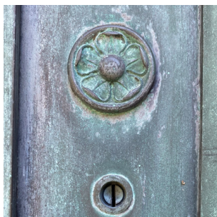
ELEMENT: DOOR CONDITION: CORROSION AND OXITATION
