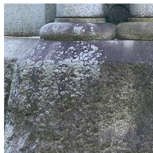
ELEMENT: PILASTER BASE CONDITION: MOISTURE / ORGANIC GROWTH
