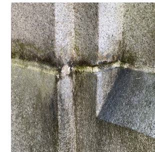
ELEMENT: JOINTS CONDITION: ORGANIC GROWTH AND EROTION
