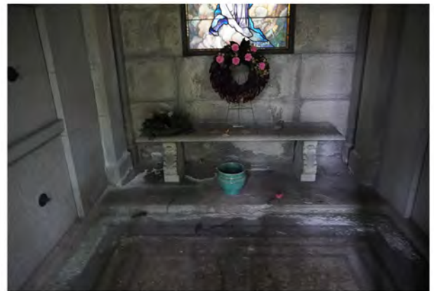
9. Interior stone salt damage1
