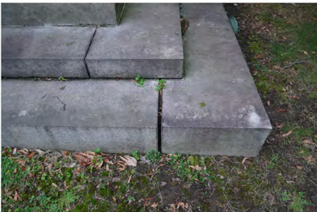
8. Gaps between step stones
