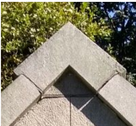
Fig. 12 The crack on the roof ridge can be seen here, extending from the sides to center
