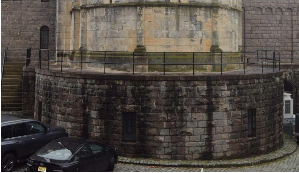
Fig.18 Pollution in the base and under the windows. Own Resource
