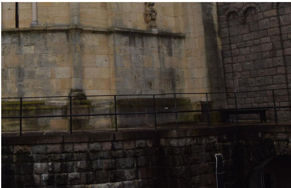
Fig.17 Water deterioration under the beading molding. Own Resource
