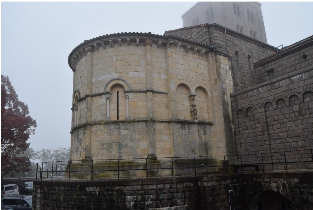
Fig.19 Biodeterioration in the upper level and under the windows. Own Resource
