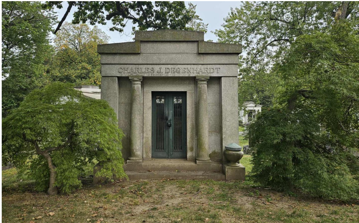
Image 15. The front façade of the Degenhardt Mausoleum with the two Japanese maple trees before it. What needs to be pointed out in this photo is evidence of rising damp and biological growth at the structure's base. One possible explanation for these conditions is the front façade's proximity to trees and the bigger trees outside of the photo's frame act as accidental shades for this portion of the mausoleum.
