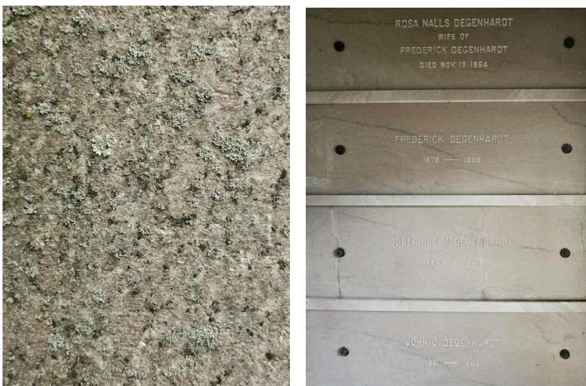
Images 16 and 17. (from left to right) - Image 16 – Close up of exterior masonry with obvious signs of biological grown. Image 17- Two vertical cracks running the entire width of the masonry face, are seen on the tombstone of Josephine Degenhardt. Up to this day, the break-in which caused the damage, has not yet been solved.
