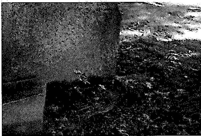
Figure 12: Root growth on the north elevation.
