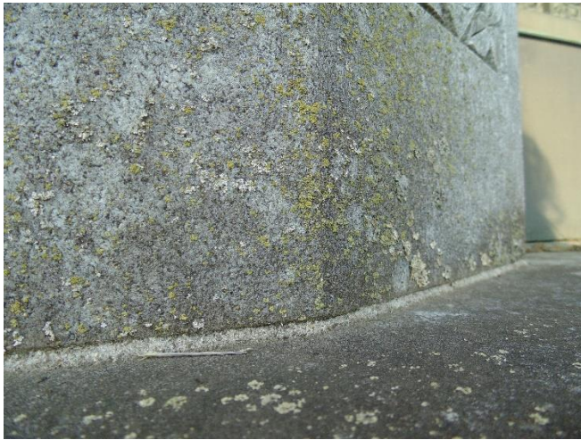
Figure 13: Detail → Biological Growth
