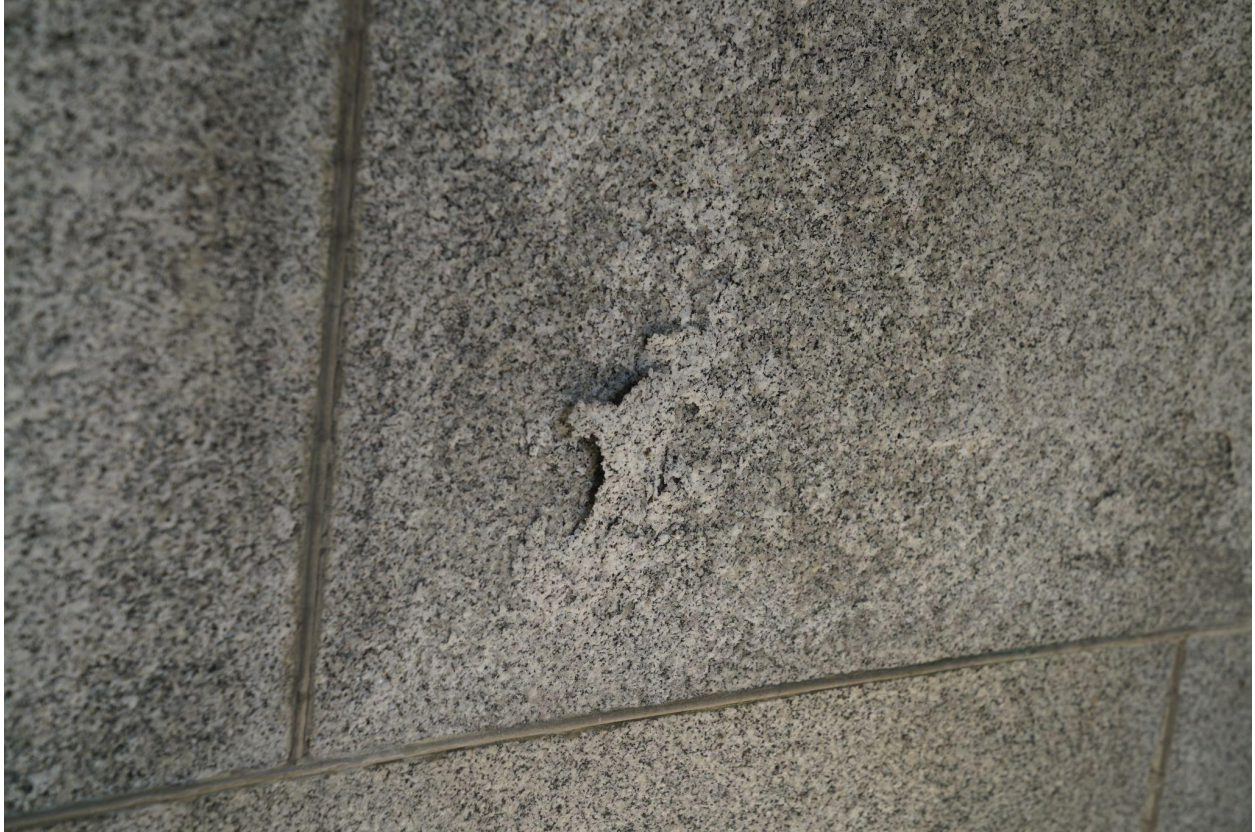
Figure 4- Blistering and flaking on the granite below the window of the mausoleum due to moisture damage.
