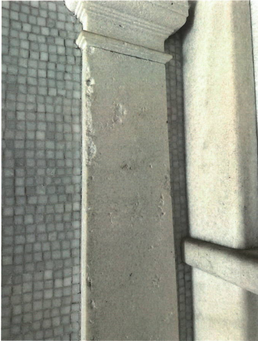
Figure 16: Santana-Miranda, Spalling of marble pilaster next to the catacombs , 2022.
