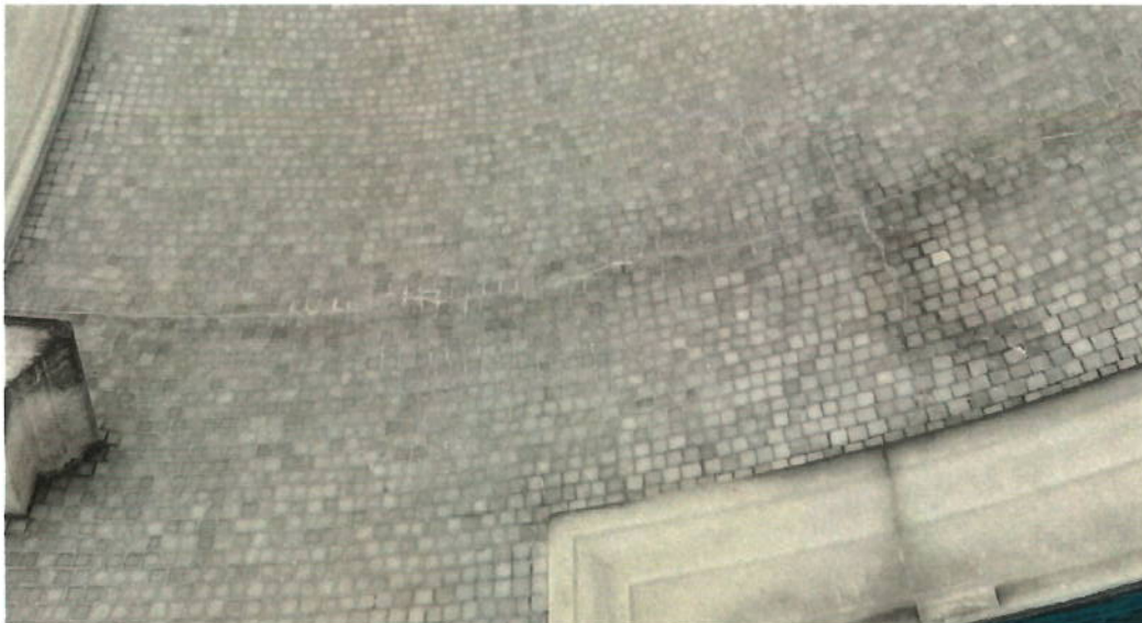
Figure 13: Santana-Miranda, Cracks in mosaics , 2022.
