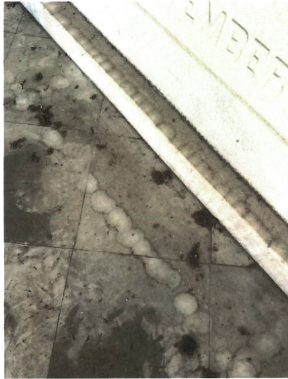
Figure 14: Santana-Miranda, Evidence of water filtration , 2022.
