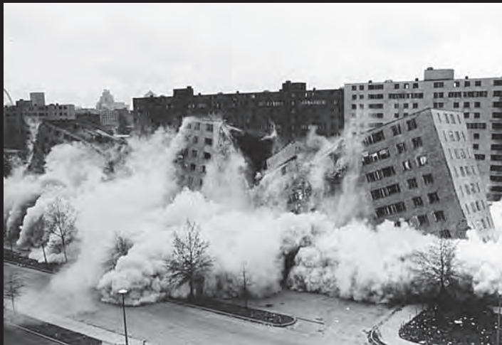
The demolition of Pruitt Igoe Houses, St. Louis, MO, 1972, Associated Press , April 21, 1972
