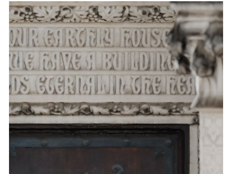
Bay 4 Close Up Detail
