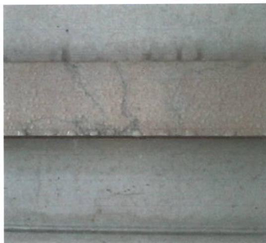
Image 12: condensation on interior
