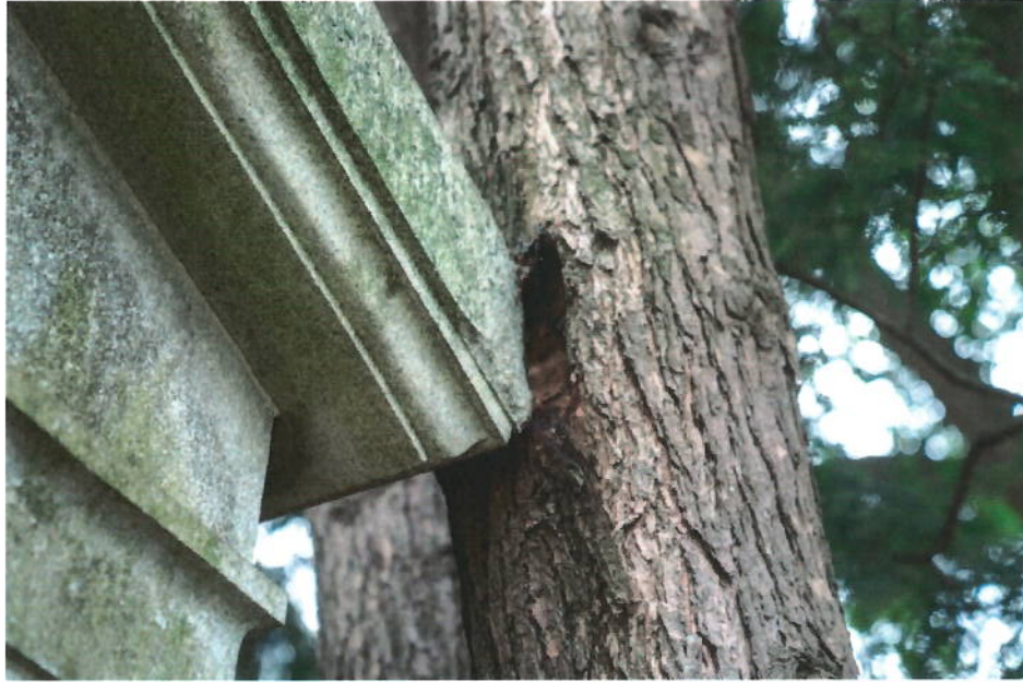
Figure 9: Phetteplace, Damaged northwest roof corner due to tree growth , 2022.
