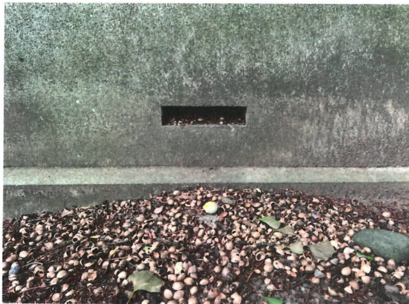
Figure 7: Phetteplace, Missing vent cover and evidence of animal interaction , 2022.
