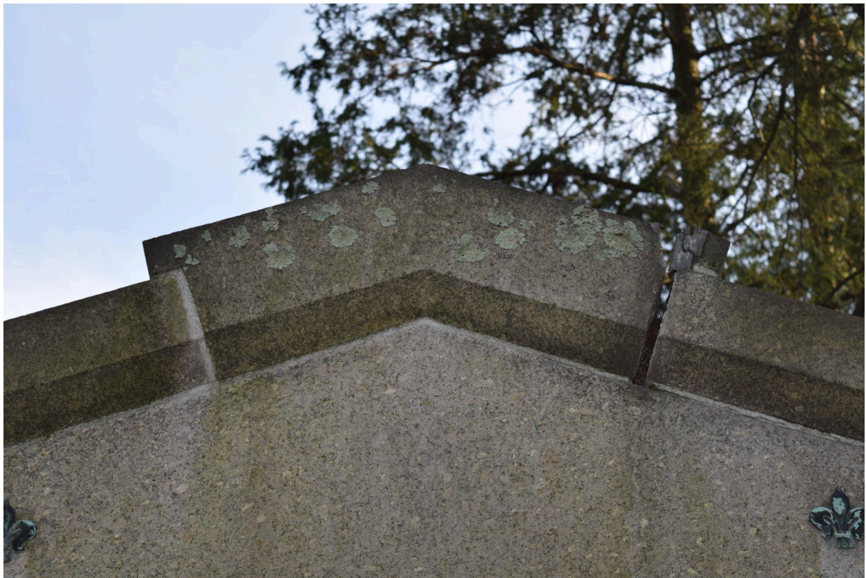
Fig. 7: Biological Growth on North Elevation
