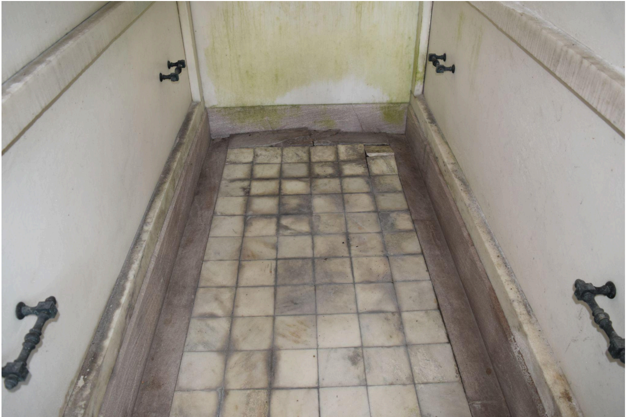
Fig. 12: North End of Interior, Showing Raised Tiles, Biological Growth, and Staining
