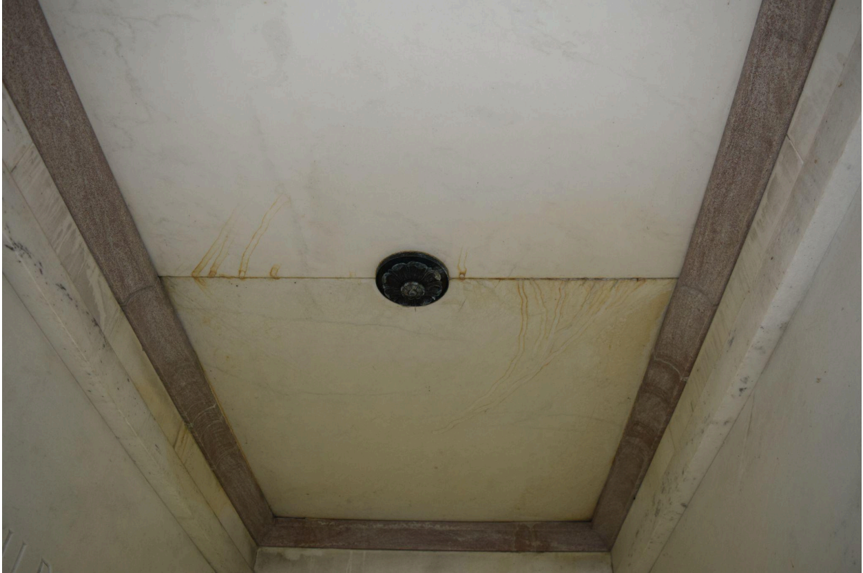
Fig. 13: Water Ingress Near Bronze Support
