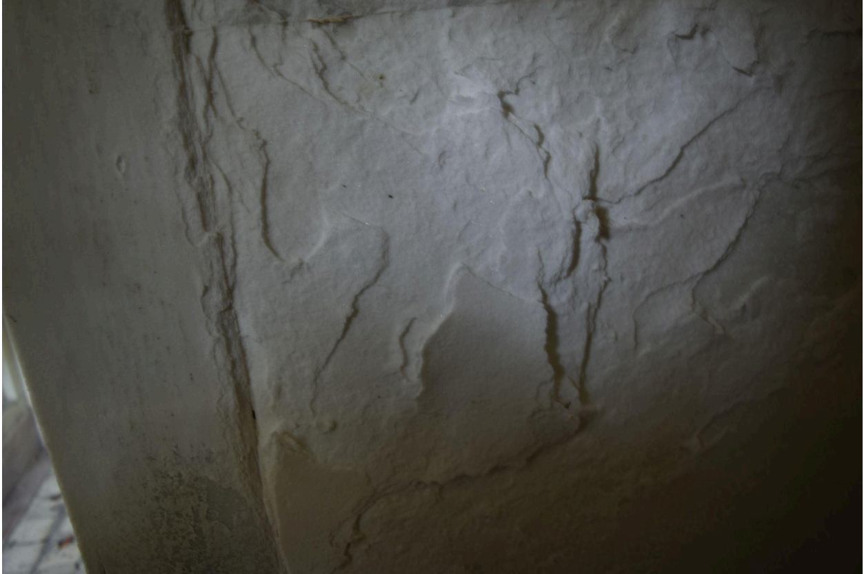
Fig. 11: Severe Exfoliation of Marble on Eastern Niches, Near Door
