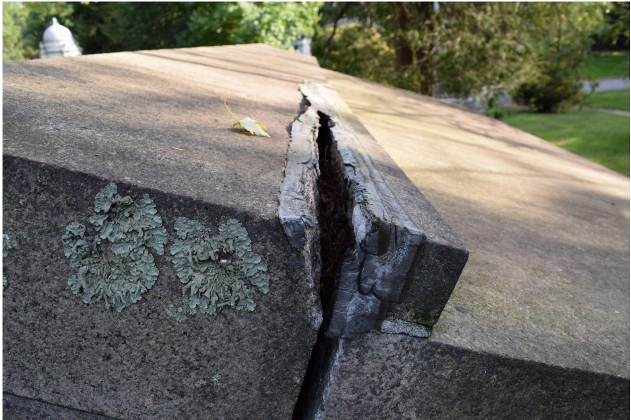
Fig. 9: Large Crack on North Elevation
