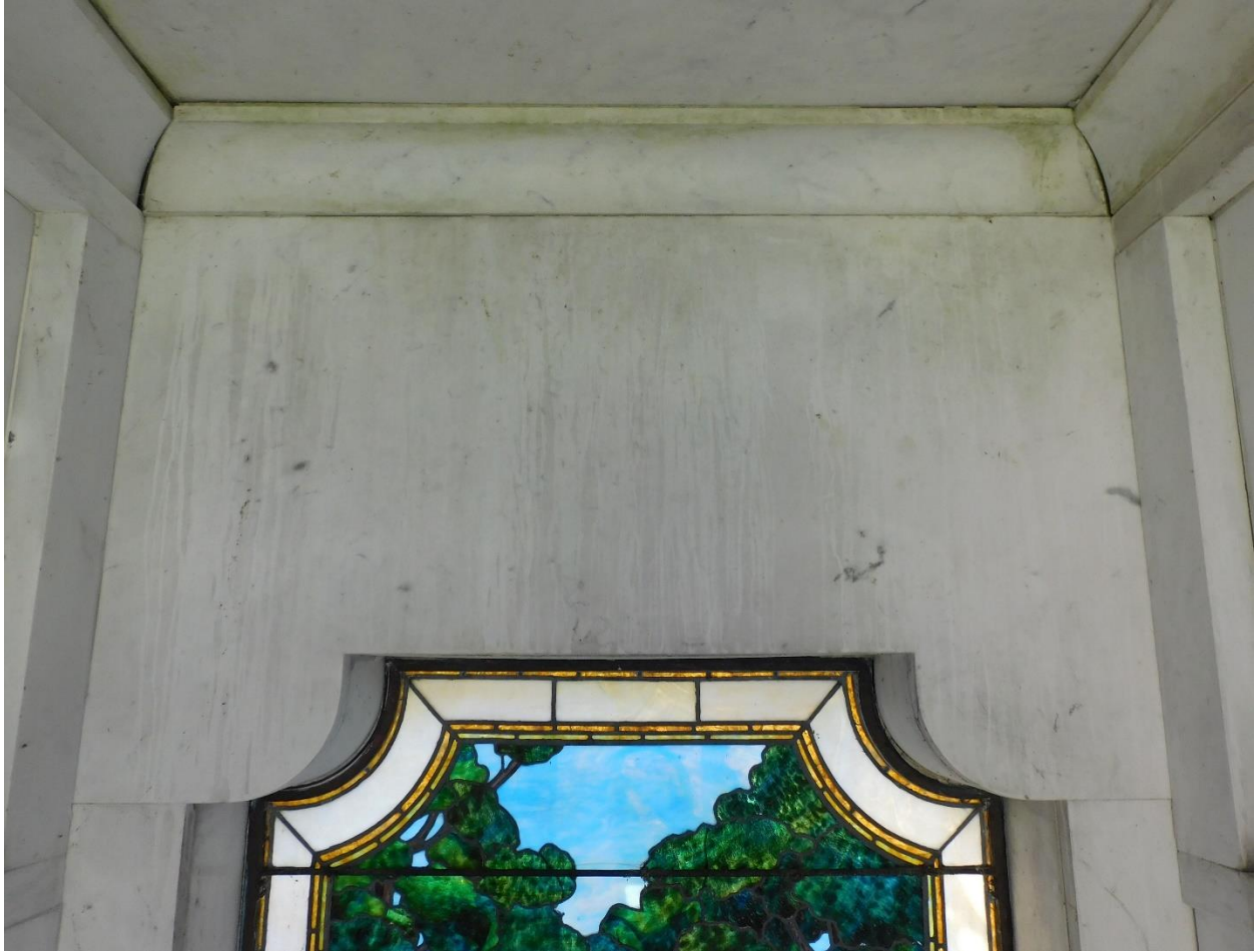
Figure 9: Conditions Detail 3, water staining and hysteresis
