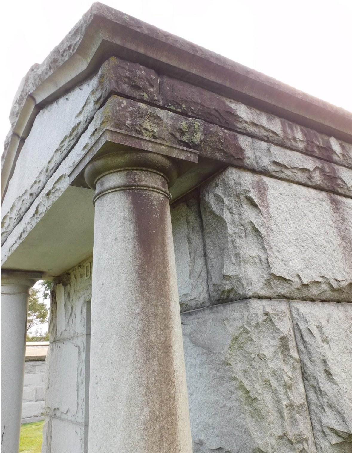
Figure 8: Conditions Detail 2, exterior biological growth
