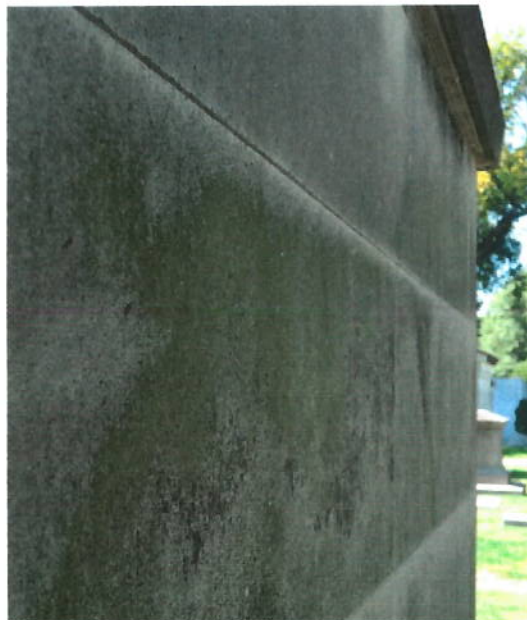
(Figure 7. West Facade, Biological Growth, Carrington Mausoleum, Woodlawn Cemetery)
