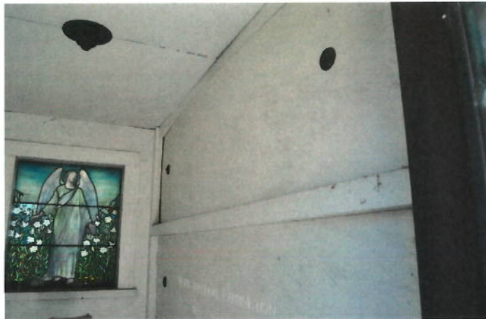
(Figure 2. Bending of Marble Slab inside Carrington Mausoleum, Woodlawn Cemetery)
