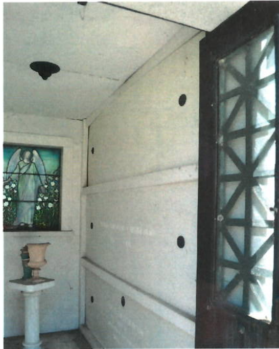
(Figure 6. Bending of Top Marble Slab Catacomb Cover, Carrington Mausoleum, Woodlawn Cemetery, 2022)
