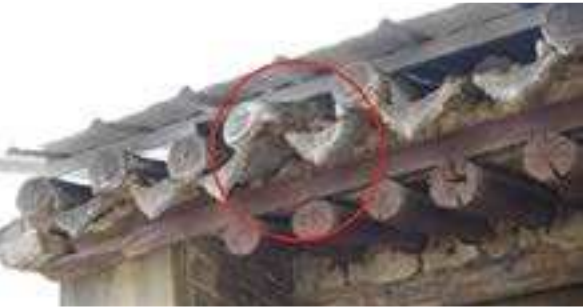
The roof tiles are loose, cracked, and missing.
