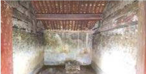
The indoor ground is damp. Below the murals on the rear wall, there was originally an altar, which is now missing.
