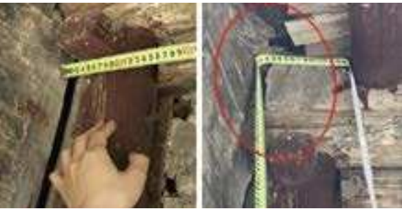
The roof tiles are loose, cracked, and missing. The tilting of the beams and walls has worsened
