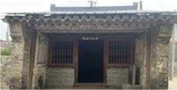
Photo of the South Elevation The building's beams and walls are tilting.
