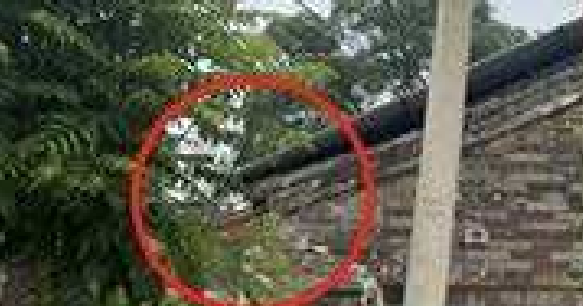
Photo of the West Elevation New through cracks have appeared on the west gable wall.
