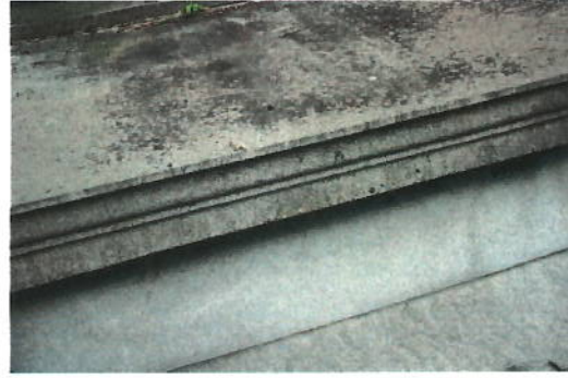
Figure 7 Frost-thaw Cycles, Photographed by W. Sun.
