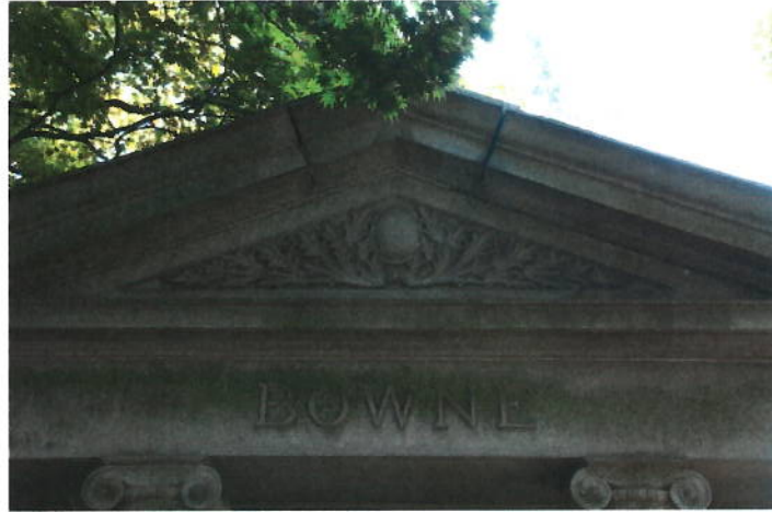
Figure 5 Mortar damage, Photographed by W. Sun.
