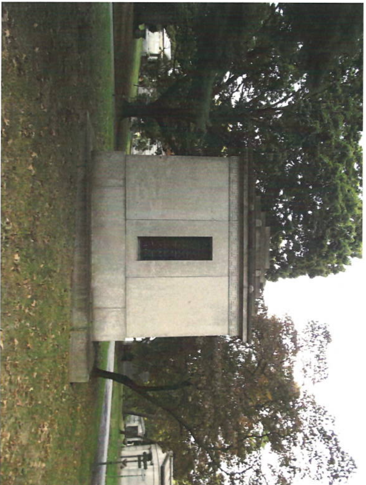
Above: Photo of rear façade showing size of granite slabs and mortar joints (img. 8)
