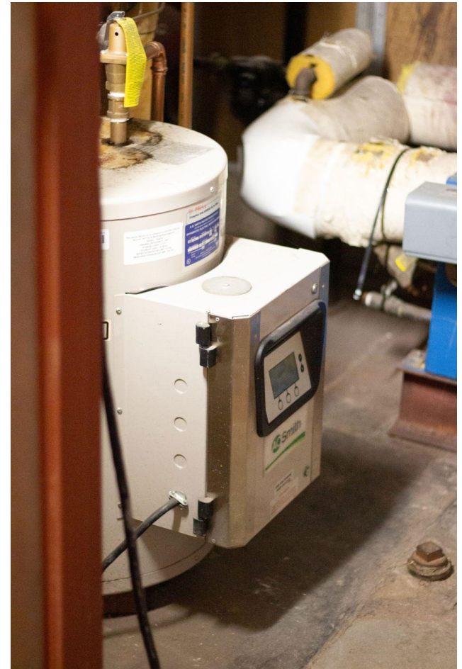
DOMESTIC HOT WATER HEATER
