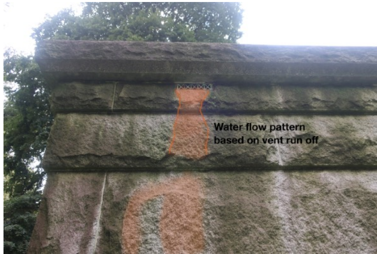
Fig. 12: Water run off path highlighted from top east vent (near south elevation).
