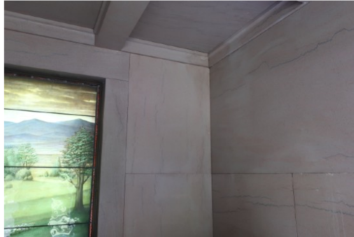
Fig. 13: Water spots on the interior cladding.
