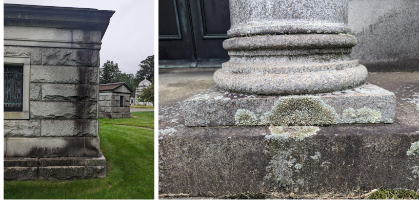
Left: staining on western facade, right: biological growth on on front facade columns
