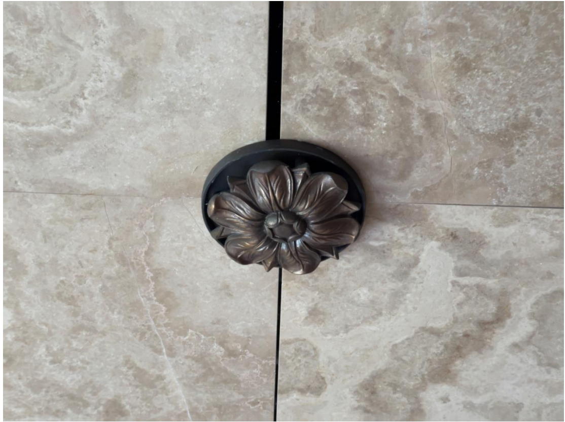
Figure 9: A marble ceiling gap. Source: Author
