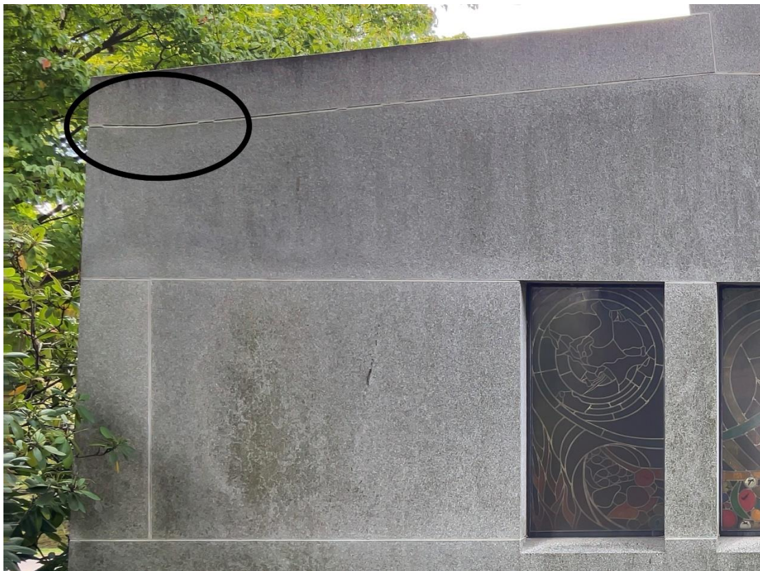
Figure 8: A crack of joint. Source: Author
