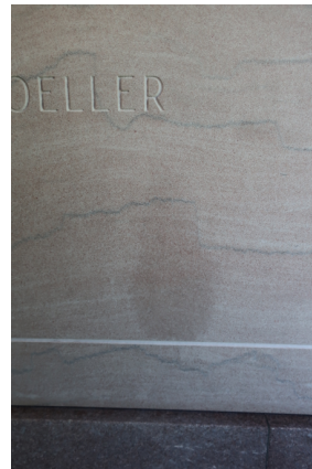
Detail: Discoloration, Essig-Foeller Mausoleum
