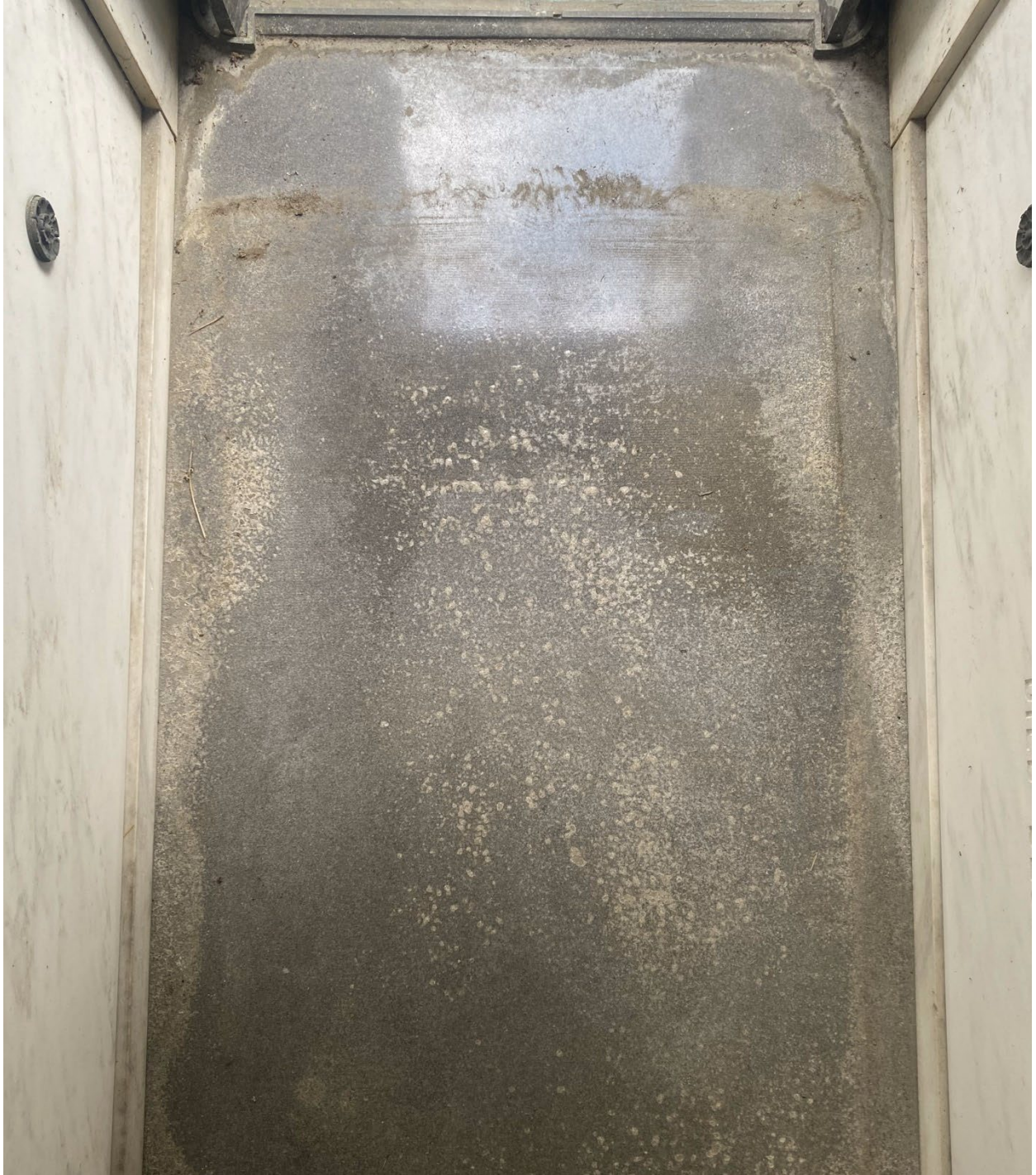
Fig. 6: Damage to finish on interior floors
